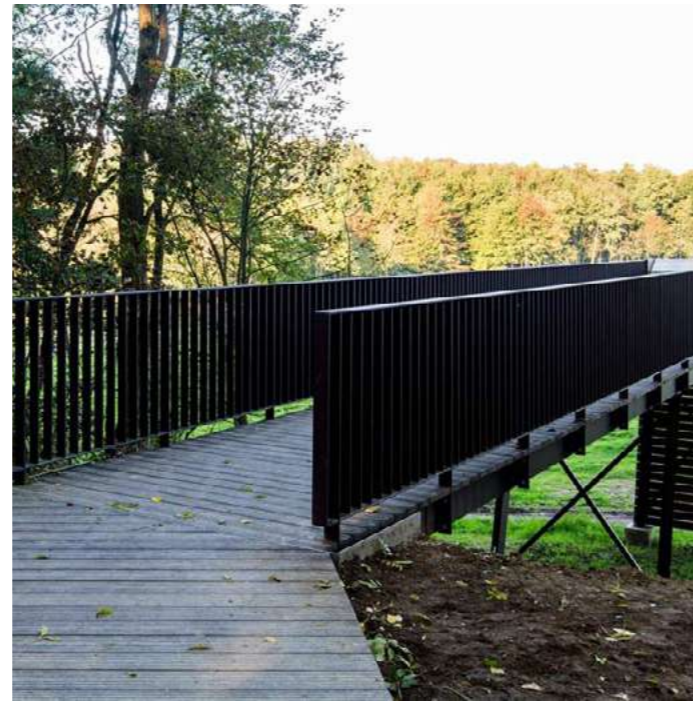
Example image: new guard and balustrade for a minor path extension to improve accessibility
